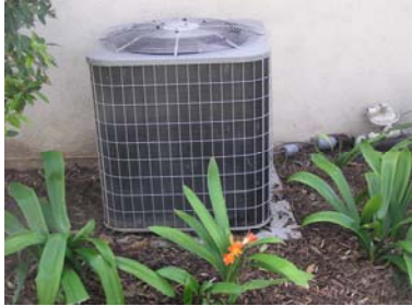
Central AC condenser
