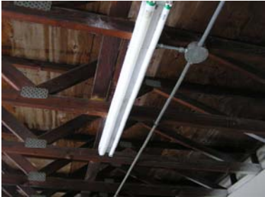
Garage lights installed incorrectly
