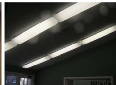
Office lights – T12 fluorescent
