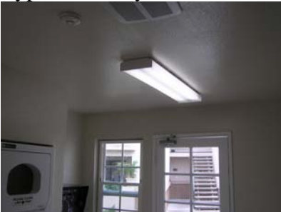
Typical laundry fluorescent fixture
