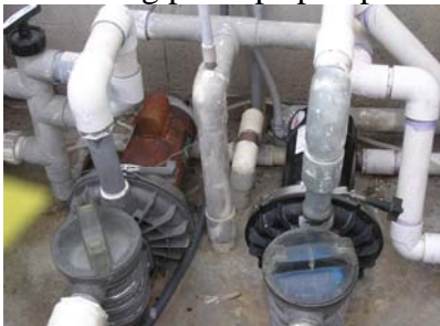
Swimming pool/spa pumps
