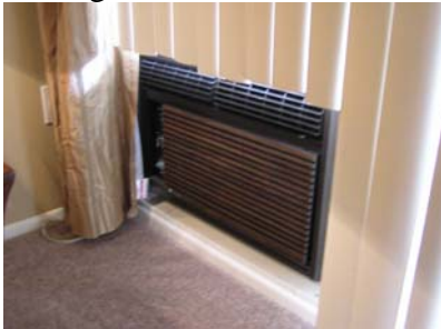
Package terminal units
