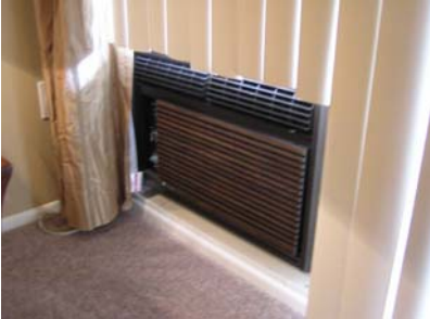
Package terminal units
