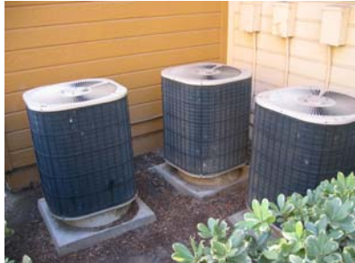
Central AC condensing units
