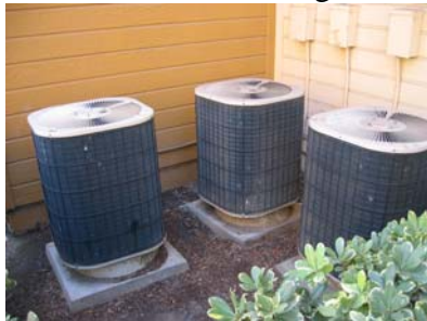
Central AC condensing units
