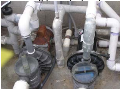
Swimming pool/spa pumps
