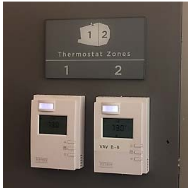
Figure 8. Thermostat Controls in the Gates-Thomas Building
